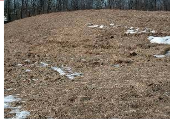
Grass mulching is applied to stabilize exposed soils and to reduce storm water runoff velocity.
